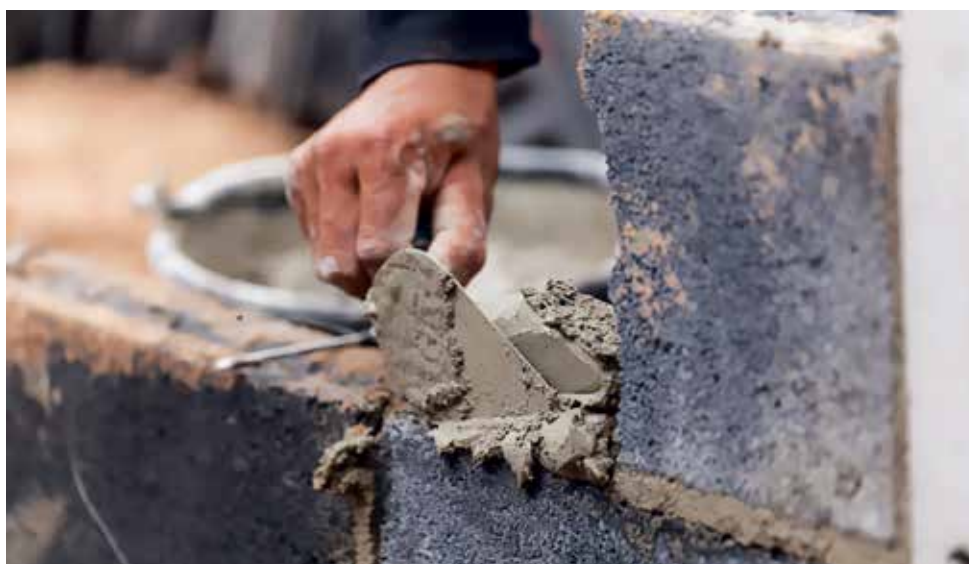
Bricklayer putting down another row of bricks in site Photo by Naypong depositphotos.com
